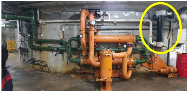
Gambar 5 Oil Vapor Discharge Pipe
