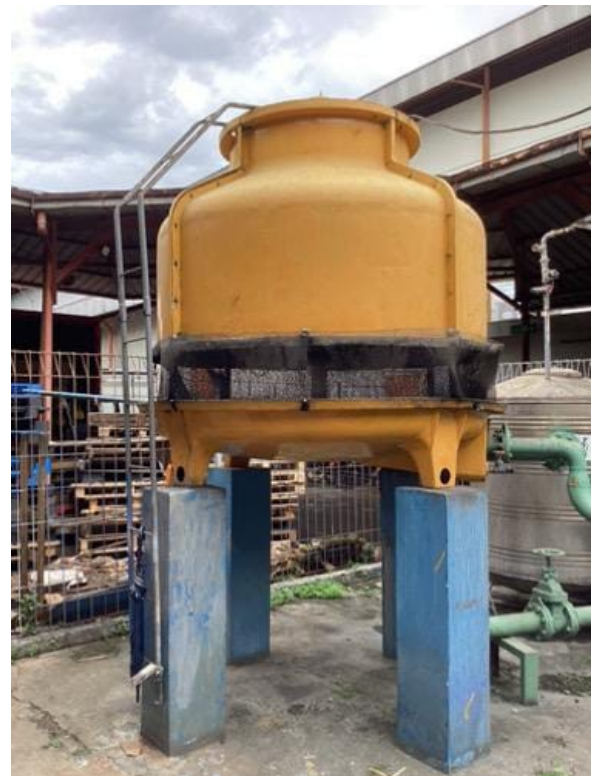
Figure 1: Cooling tower in PT. XYZ
