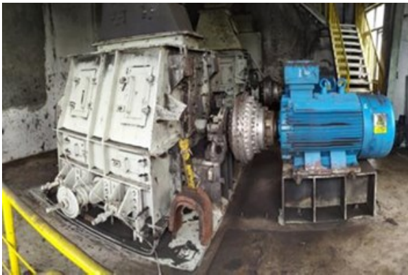
Figure 1: Motor and Coal Crusher
