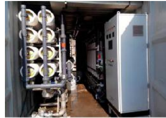
Fig. 3. Installation Reverse Osmosis Process
