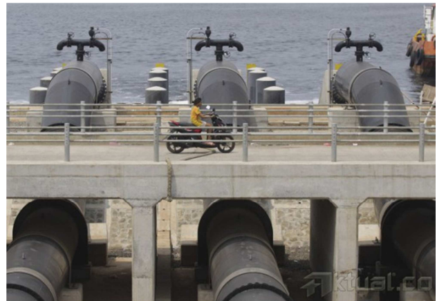
Figure.1.17: An example of flood prevention water pumping station in DKI Jakarta [DKI Jakarta]
