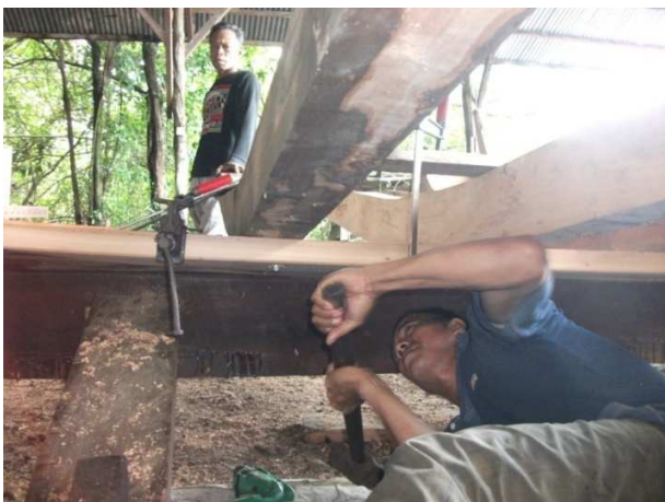
Figure 10: Unsafe condition when planking.
