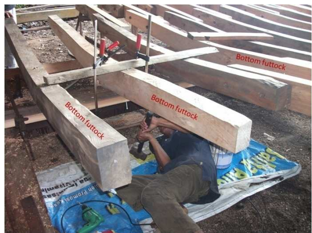
Figure 8: Unsafe condition when hitting a nail in the keel
