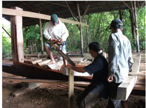
Figure 7: Unsafe condition when cutting the wood.
