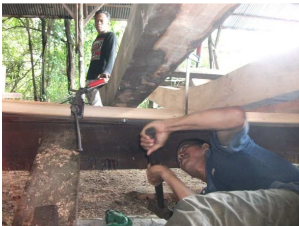
Figure 10: Unsafe condition when planking.
