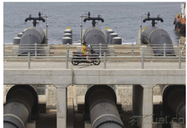
Figure.1.18: An example of flood prevention water pumping station in DKI Jakarta [DKI Jakarta]
