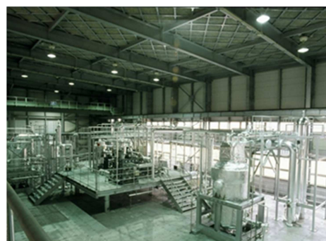
Figure 3: 30 kW OTEC and Desalination Room, Saga-Japan [IOES]
